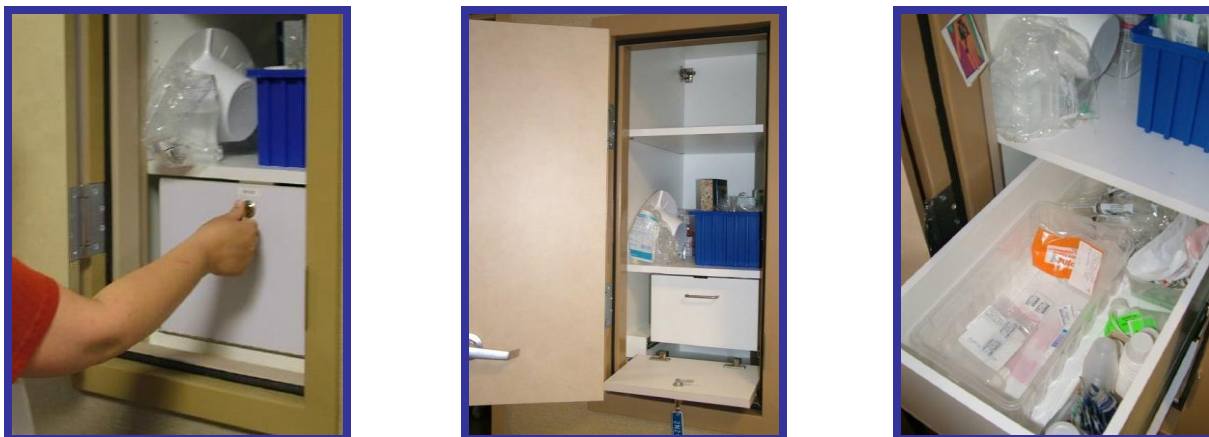
View of patient servers from the hallway.
